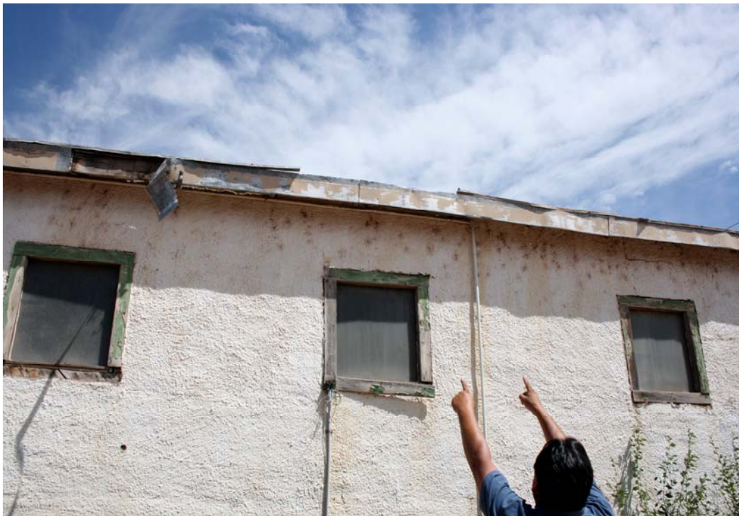
Station was located on roof of building on a small platform.
